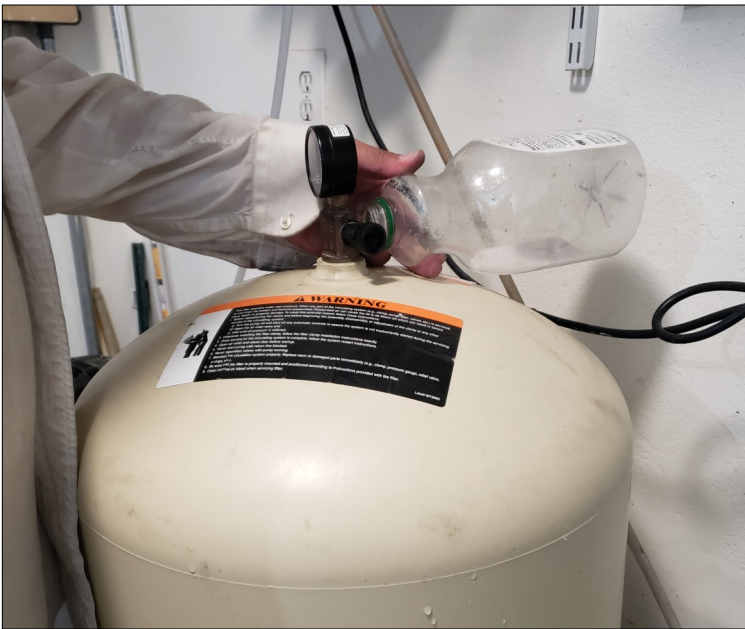
Recycling and keeping the walls dry. Pool tech uses empty plastic bottle after releasing air to catch the water.
